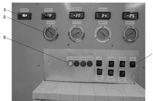
Figure 3 Display and control panel (1-Thermometers 2-Pressure gauges 3-Indicator lights 4-Control switches).
